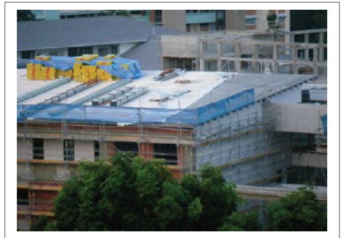
Figure 4. Picture of a construction site where the Spectrum 3 can be used to determine the correct side of single coated glass to be installed.
